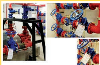
Fixed Fire Pump Room
