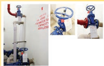
Fire Services Transfer Pumps and Tank
