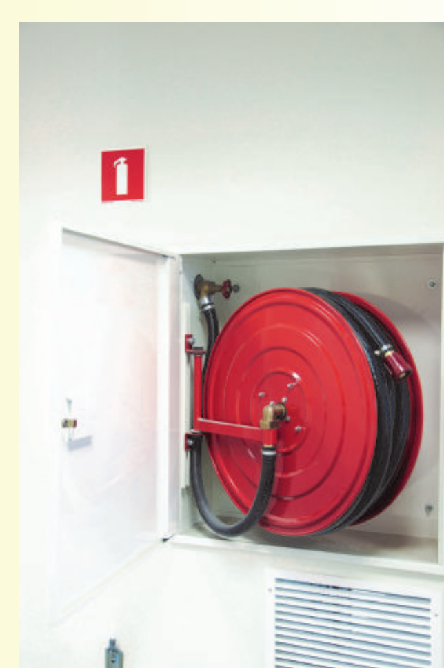
Fire Hydrant / Hose Reel System
