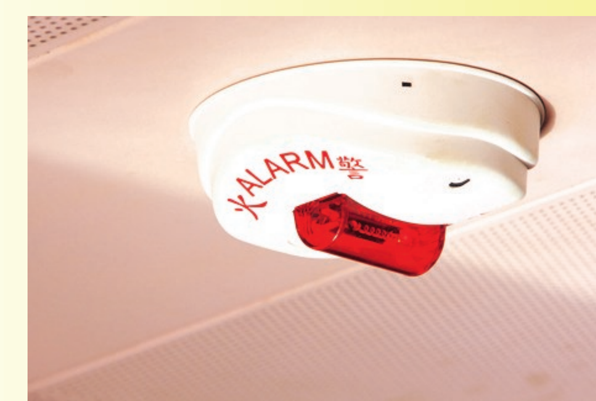
Visual Fire Alarm
